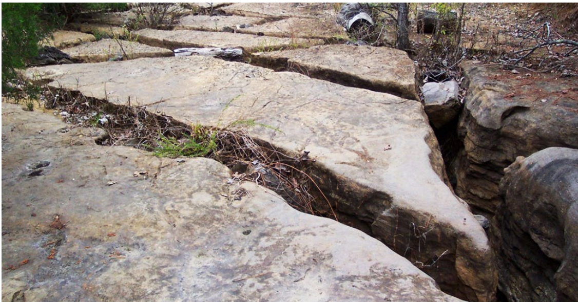
Figure 3. Close-up view of solution channels along joints in the basal limestone of the Green Hill Member below the spillway, seen at top, of Haynes Lake in Tishomingo State Park. Picture (digital; Image 835) taken by Stephen Jennings on November 7, 2003.
